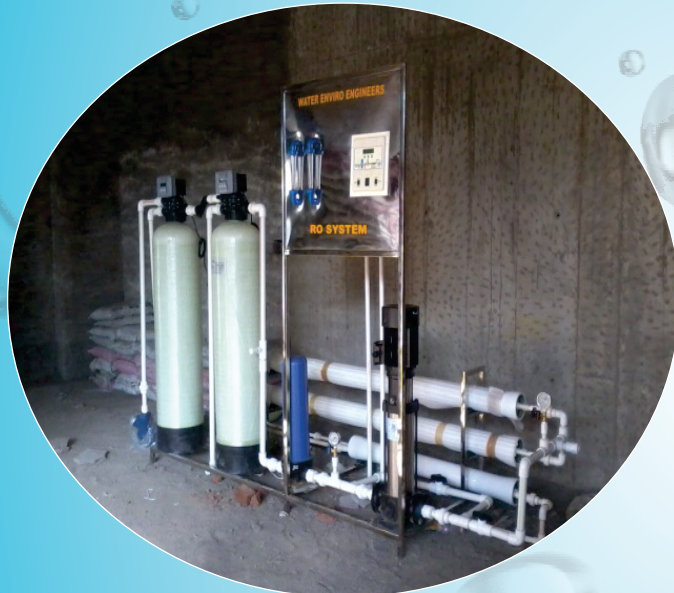
Reverse Osmosis Plant
