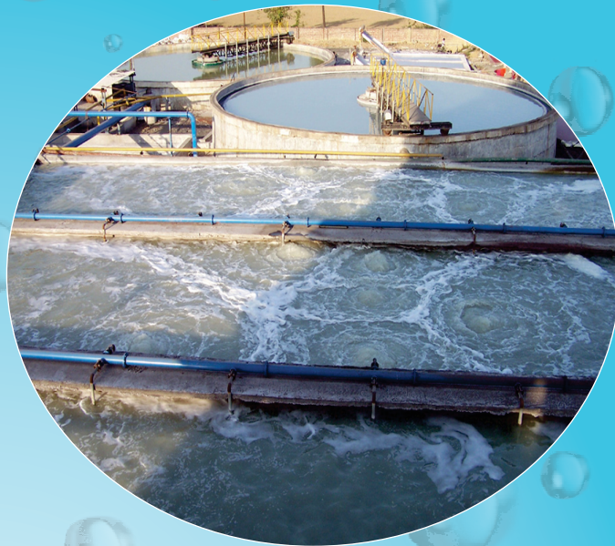
Effluent Treatment Plant
